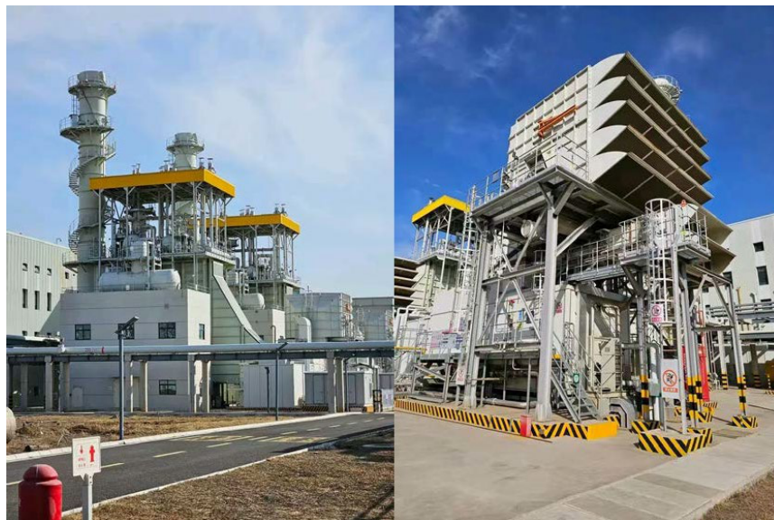
Siemens SGT-700 1×1 Combined Cycle Plant — As Installed
