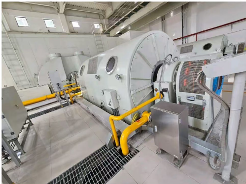
Steam Turbine Generator 12 MW Dongfang STG in the turbine hall
